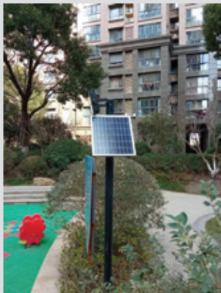
Solar lighting set up on pavement and lawns inside the community 在園區道路及草坪設置太陽能照明燈
