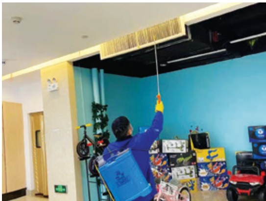
Disinfecting the air conditioning equipment 疫情期間對空調設備進行消毒
